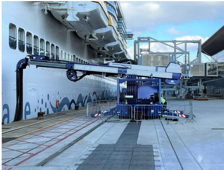
Figure 41: Shore power at Horizon Cruise Terminal 70
