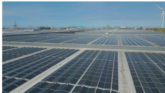
Figure 9: solar park on Patrizia buildings along Witte Zeeweg 3-21 on the Maasvlakte 20 .
