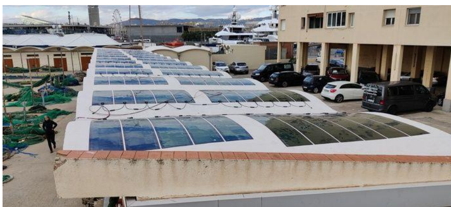
Figure 6: The Port of Barcelona plant (7 MW of solar energy)
