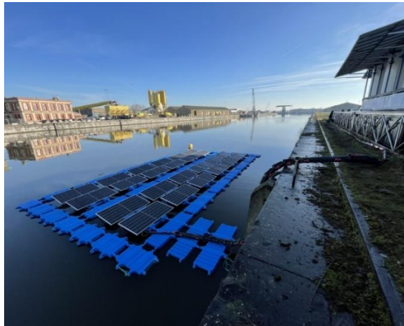
Figure 16: Floating solar power plant in Port Oostende, Belgium 31
