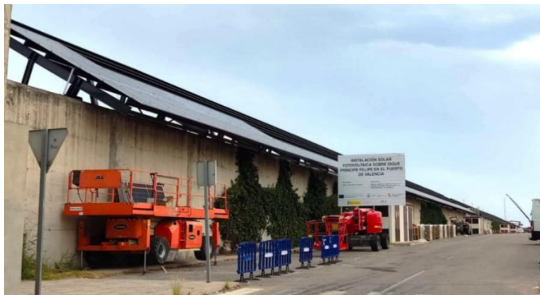
Figure 2: Installation of the photovoltaic power plant located on the Principe Felipe dock
