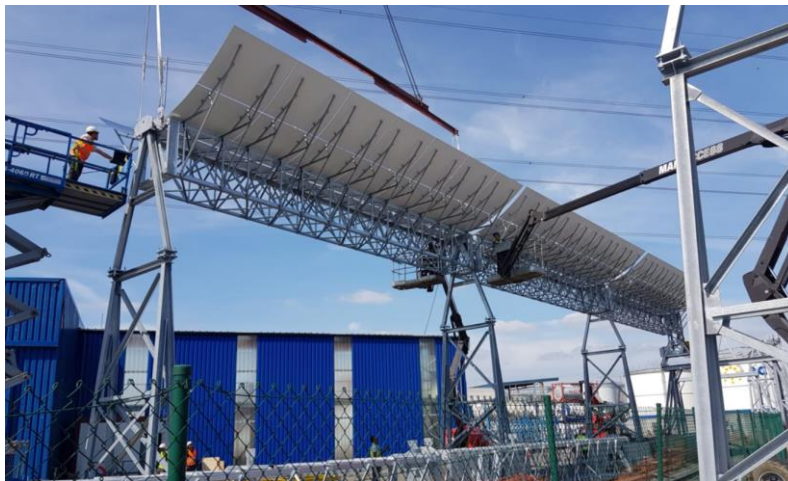
Figure 14: Concentrated Solar Thermal Energy (CST) farm in the port of Antwerp 27
