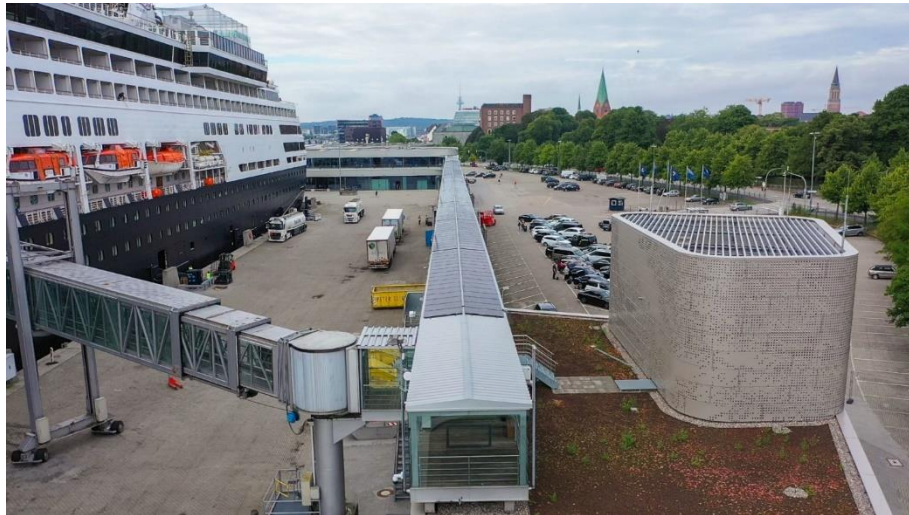
Figure 29: Photovoltaic system installed at the cruise terminal 50
