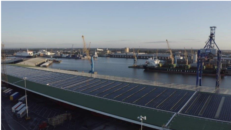
Figure 39: Rooftop solar array in the port of Hull 68
