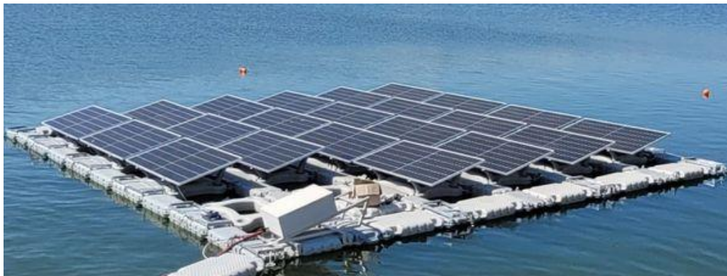
Figure 24: Unique floating PV energy production project in Constanța Port 41
